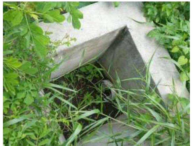
Borehole BHD site at Overland Magnum. Closer view of concrete catchment or energy dissipator with entry and exit pvc pipes. Chamber will collect and allow some settling of water to reduce turbidity as well as reduce velocity before being released into river.
