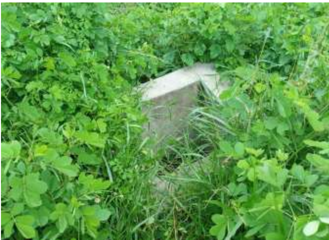
Borehole BHD site at Overland Magnum. Concrete catchment pit constructed to capture runoff from overflowing waters from the previous borehole exercise. This is a control to reduce the effects of scouring and degrading the land in an uncontrolled manner.
